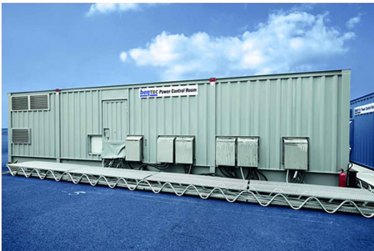
Slika 9. PCR – Power Control Room
