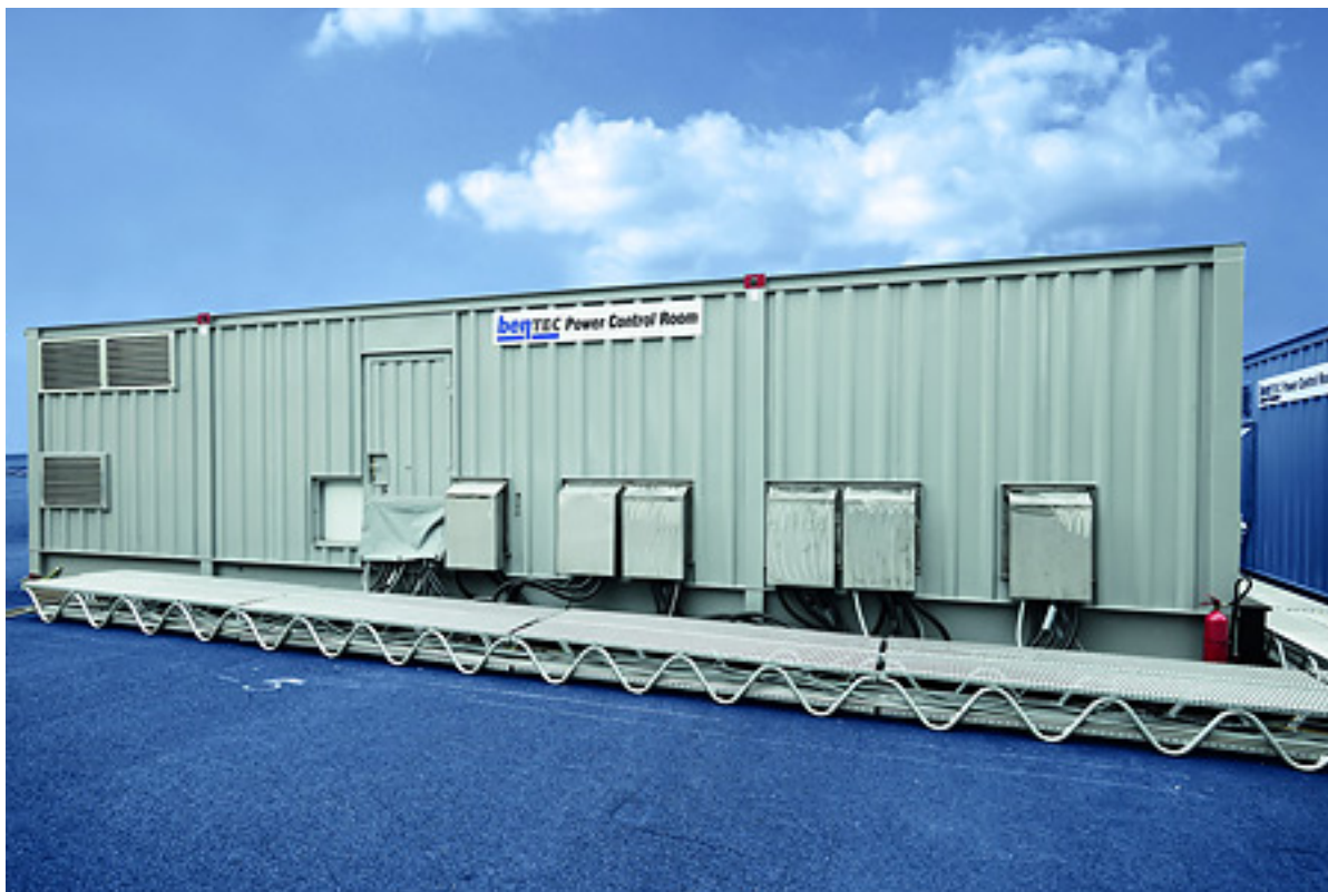
Slika 9. PCR – Power Control Room
