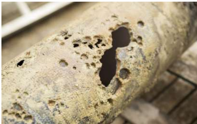
Slika 9. Primjer rupičaste(pitting) korozije ( https://www.nufLOWmidwest.com/2-types-of-corrosion-that-occur-in-industrial-piping-systems/ Pristupljeno 15.07.2021)
