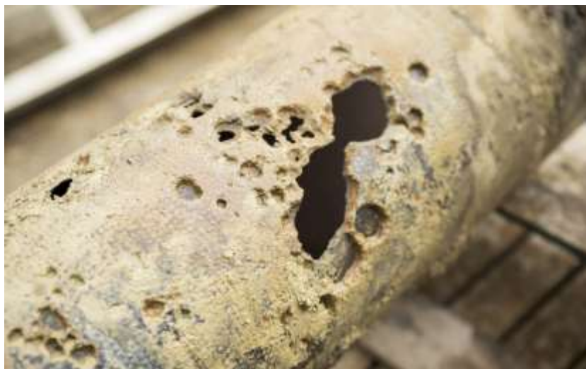
Slika 9. Primjer rupičaste(pitting) korozije ( https://www.nufLOWmidwest.com/2-types-of-corrosion-that-occur-in-industrial-piping-systems/ Pristupljeno 15.07.2021)
